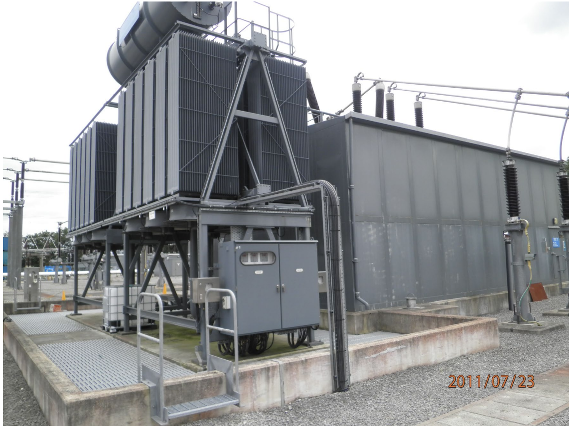
Figure 4.3: Typical (large 400kV) power transformer
