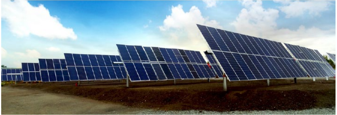
Figure 4.1: Typical tracking panels
